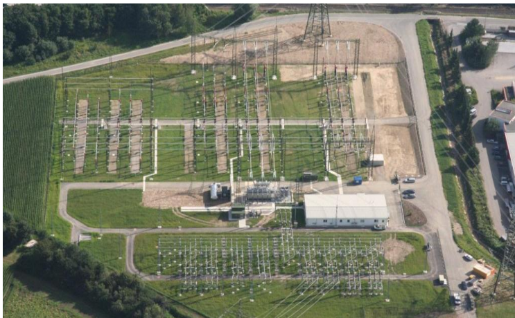
AUSTRIAN POWER GRID AG
